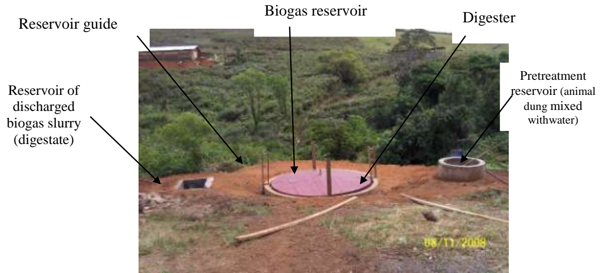
Fig.1. BIOFARM Centre floating drum biogas system built in 2008.
